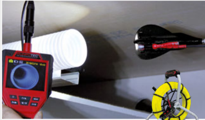
Ventilation inspection and servicing
