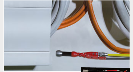
Shafts and underfloor ducting
